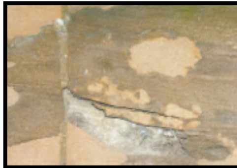
Close up of Portland Formation brownstone shows weathering caused by freeze/thaw cycle.
